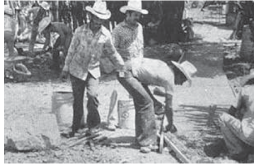
In the village of Ajoya, Mexico, over 60 families participated in building a cement walkway from the rehabilitation center to the main street.
