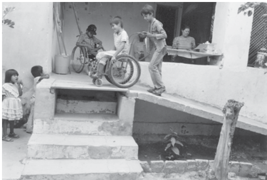
The health workers of Project Piactla built this ramp so the wheelchair riders could come into the clinic more easily. (Photo: John Fago)
