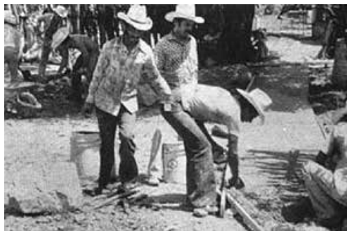
In the village of Ajoja, Mexico, over 60 families participated in building a cement walkway from the rehabilitation center to the main street.
