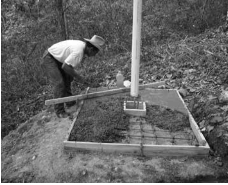
A local handyman builds a concrete latrine slab in the mountains of Honduras.
